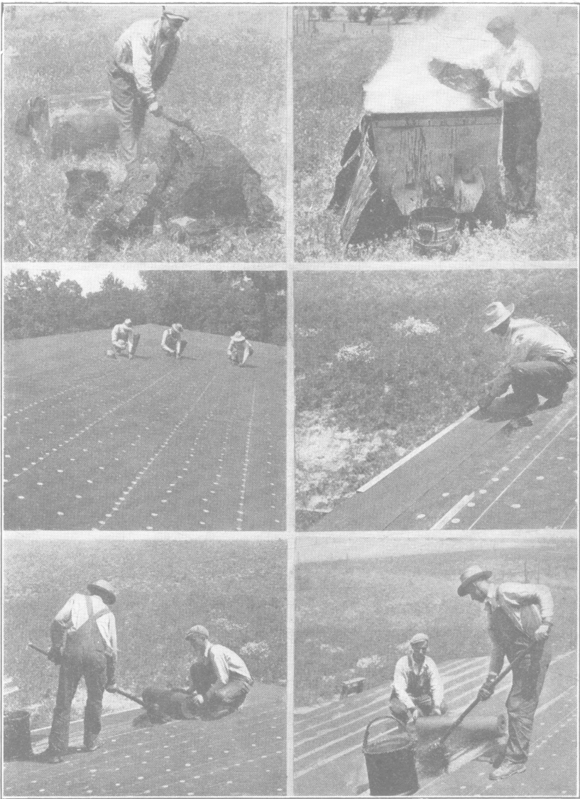
FIG. 20.—STEPS IN MAKING A BUILT-UP ROOF (Read from upper left to lower right).
