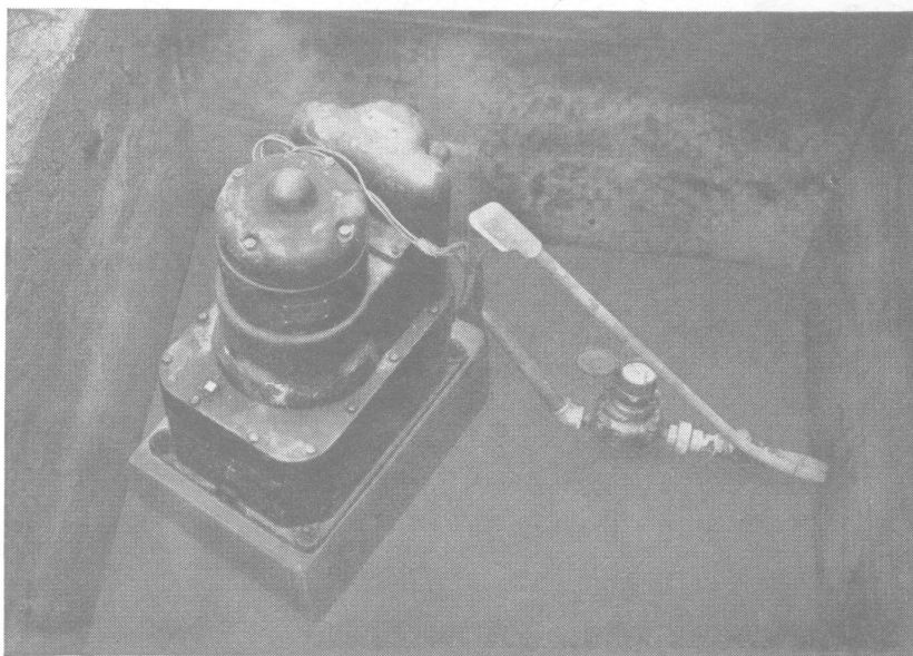
Figure 10.—All the well water for livestock and household uses is pumped by this deep-well system on George Rausch's farm. This outfit consumes 1 kw-hr. for every 575 gallons of water delivered.
