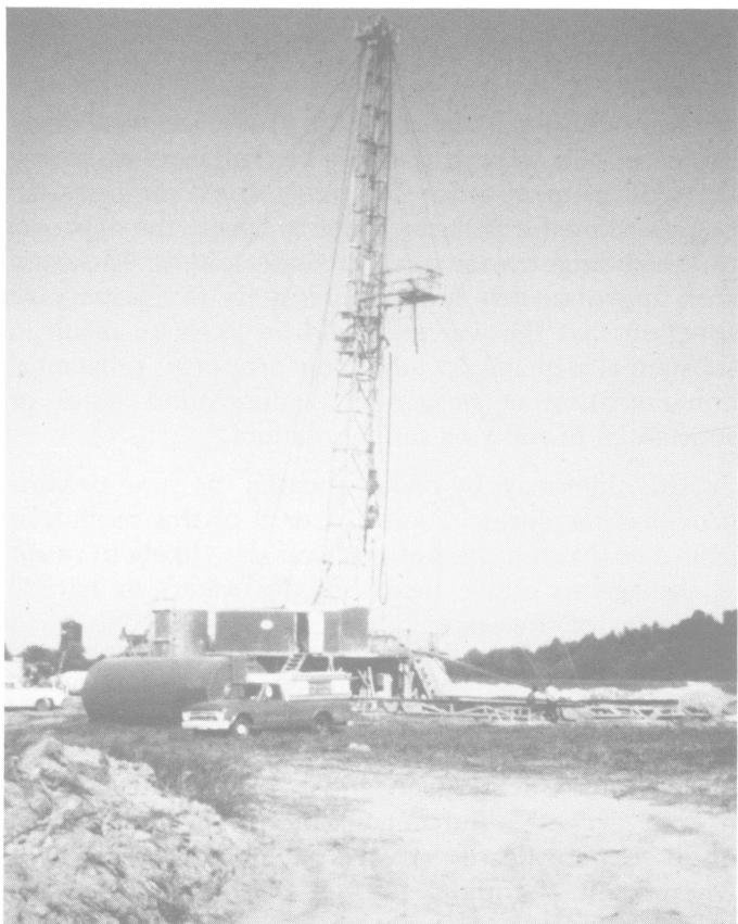
Restoration and reclamation are important lease concerns. This access road, for example, can be left on-site after production, regraded or removed — depending on provisions of the lease and addendum.
