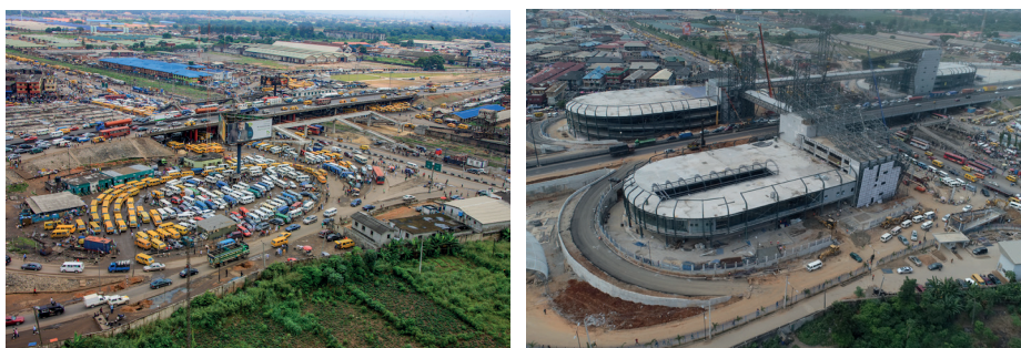
Aerial picture of the Oshodi Transport Interchange before and after new construction work. Photo credit: Planet Projects Ltd.
