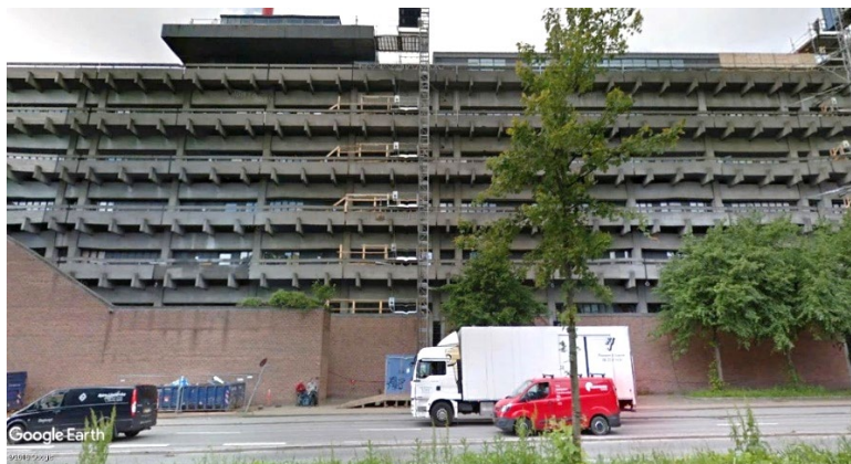
Figure 6. Refurbishment work going on at a brutalism piece of architecture in Copenhagen - the Panum Institute (1974-1976) Will the whole upper concrete part be enveloped in glass for the sake of insulation, or what will happen? Google Earth, 2019
