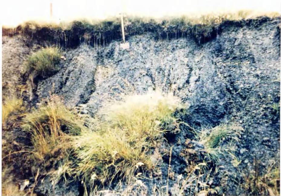
PLATE 10 - ENTERKINE - Eroded bank showing saturated soil layer.
