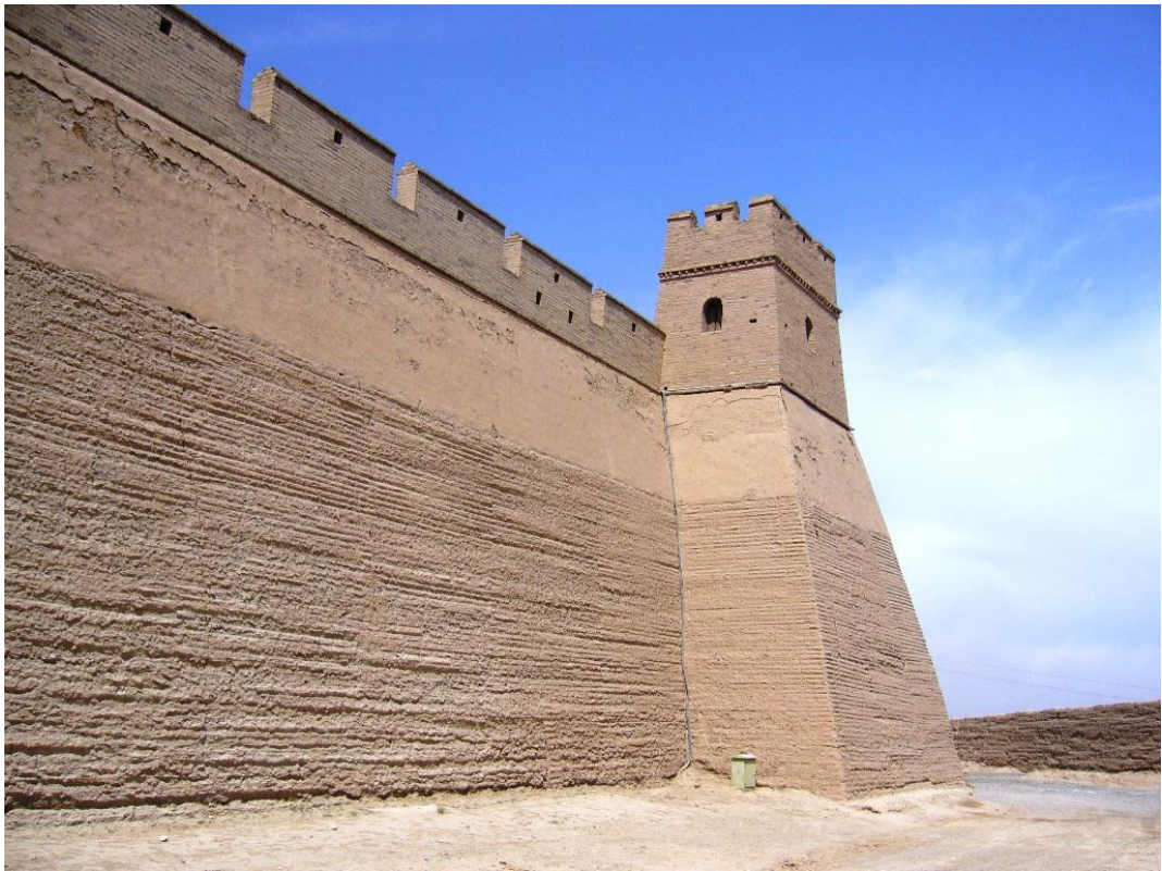
Figure 2.1. Rammed earth portion of The Great Wall of China at Gansu, China. Photo retrieved from https://www.murailledechine.com/voyage-jiayuguan-gansu
