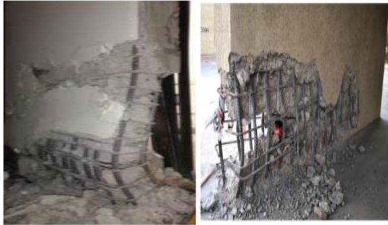
(a) (b) Figure 2.2. Failure of RC walls: (a) Chile earthquake; (b) Christchurch, New Zealand (Marius, 2013)
