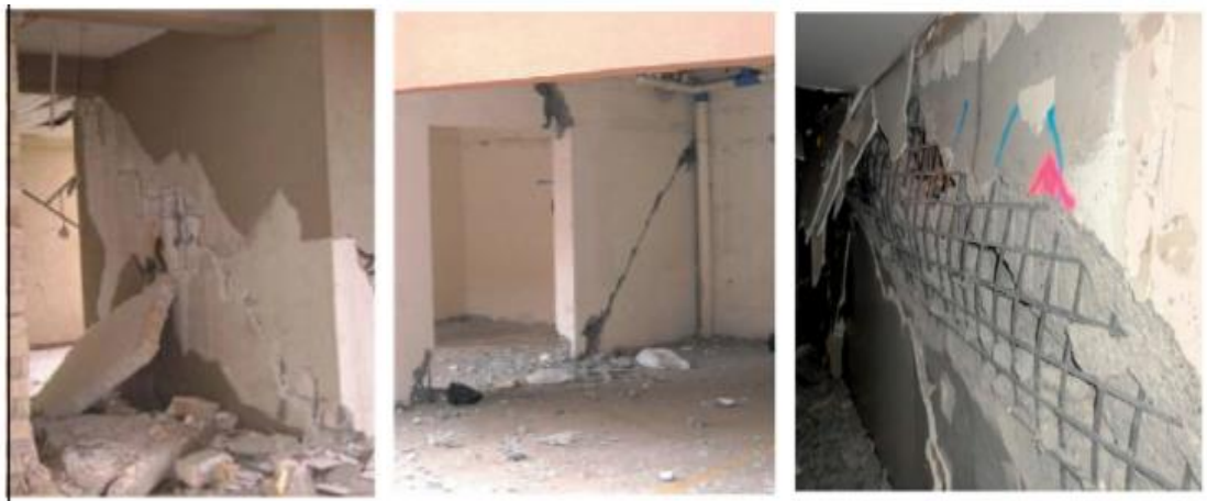
(a) (b) (c) Figure 2.3. Shear failure of RC walls: (a) L'Aquila, Italy; (b) Christchurch, New Zealand; (c) conception, Chile (Marius, 2013)
