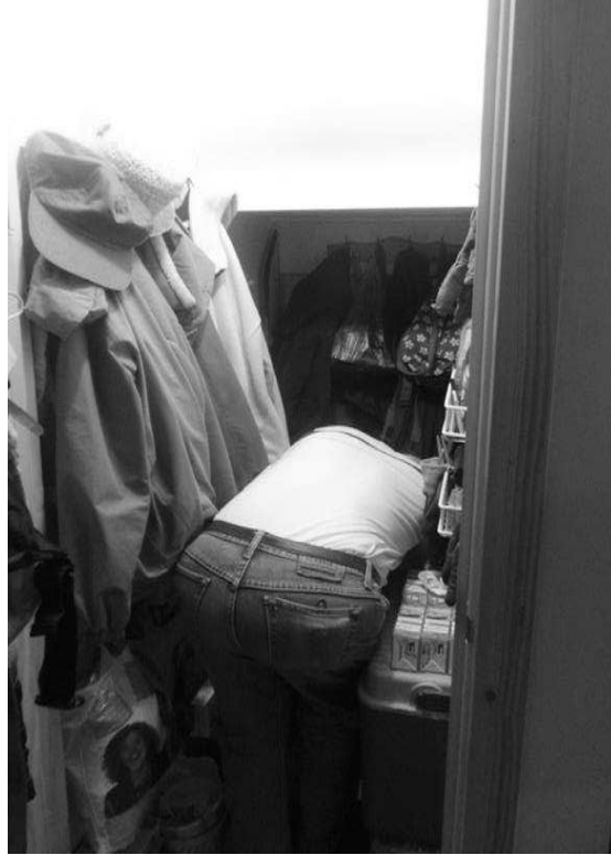
Figure 11. Poor location of the inverter (A)
