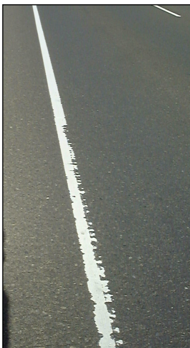
Transition from 180 mil slot backfilled with 120 mils of material (top) to a 125 mil slot backfilled with 95 mils of material (bottom).
