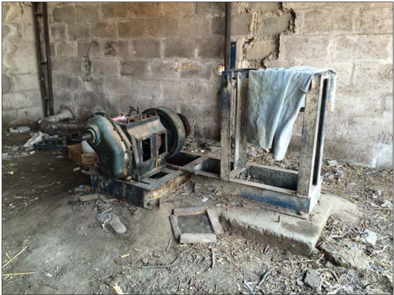
Figure 1. Broken Down Equipment
