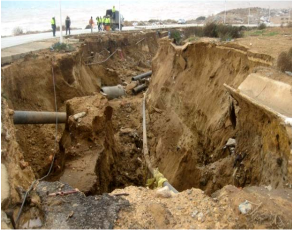
Fig. 1 – Destruction of roads and canals
