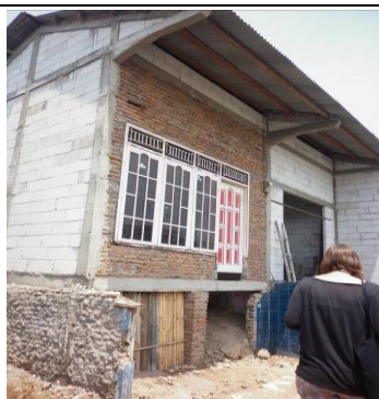
Figure 13. One of the houses to be elevated due to a decrease in soil
