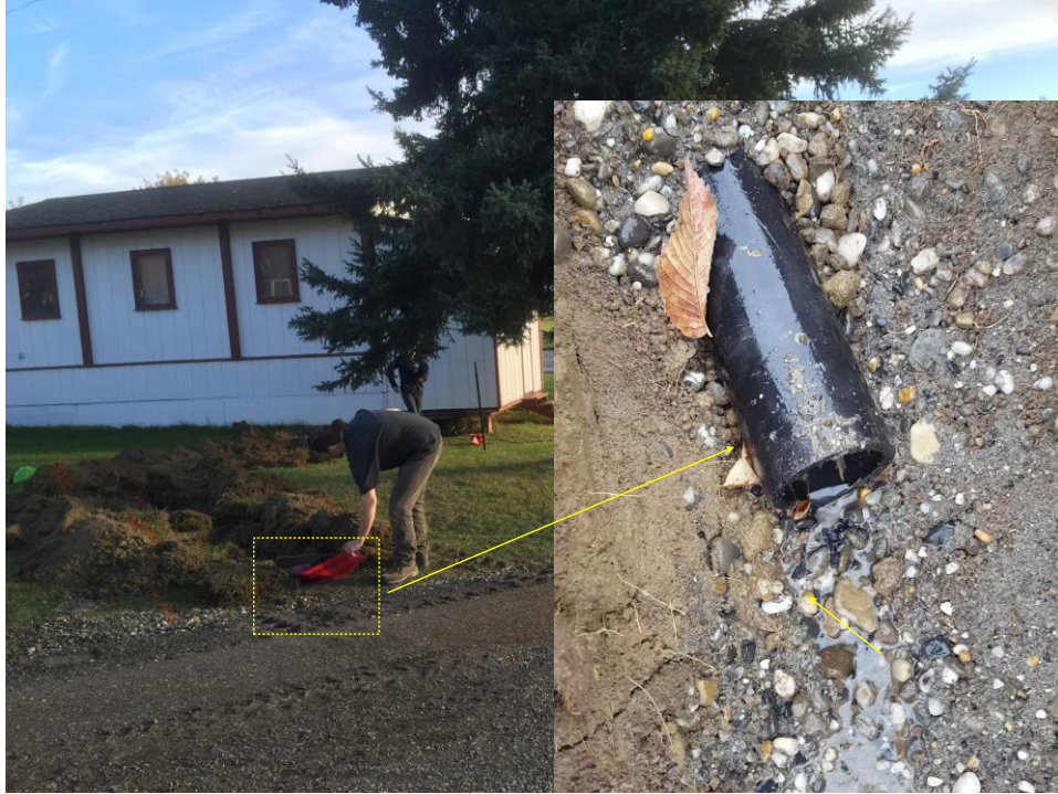
Figure 3.16 Drainage pipe outlet
