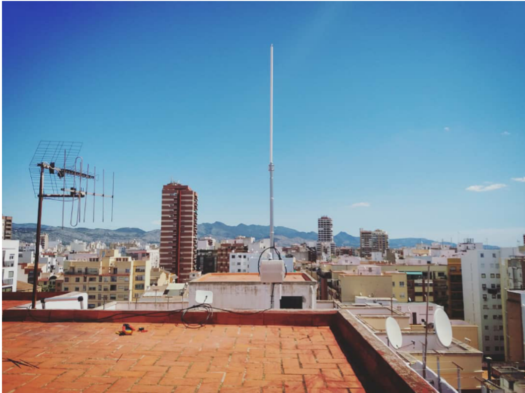
Figure 2.4: One of the gateways installed in Castellón de la Plana
