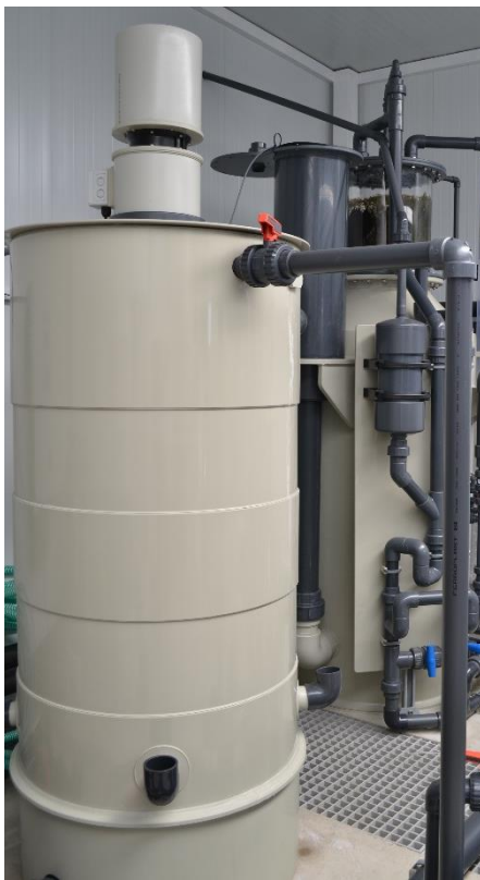
Figure 12: "Biotower", where nitrification process and carbon degassing occur. Photograph by Adriana Laranjeira, Riasearch.
