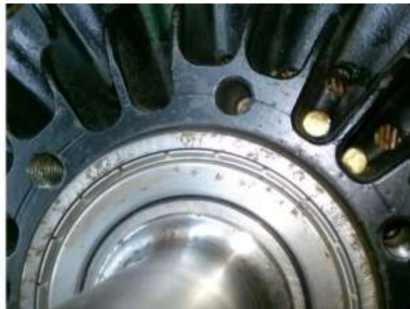
Figure 5.51 – Rust detected in the bearings and shaft
