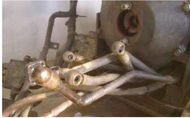
Figure 5.11 – Loose tubes after triple pumps module removal
