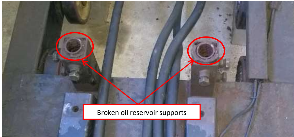
Figure 5.17 – Broken oil reservoir supports
