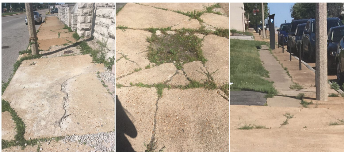
Figure 11: Photos of sidewalk conditions on Grandel Square, just west of Grand Boulevard
