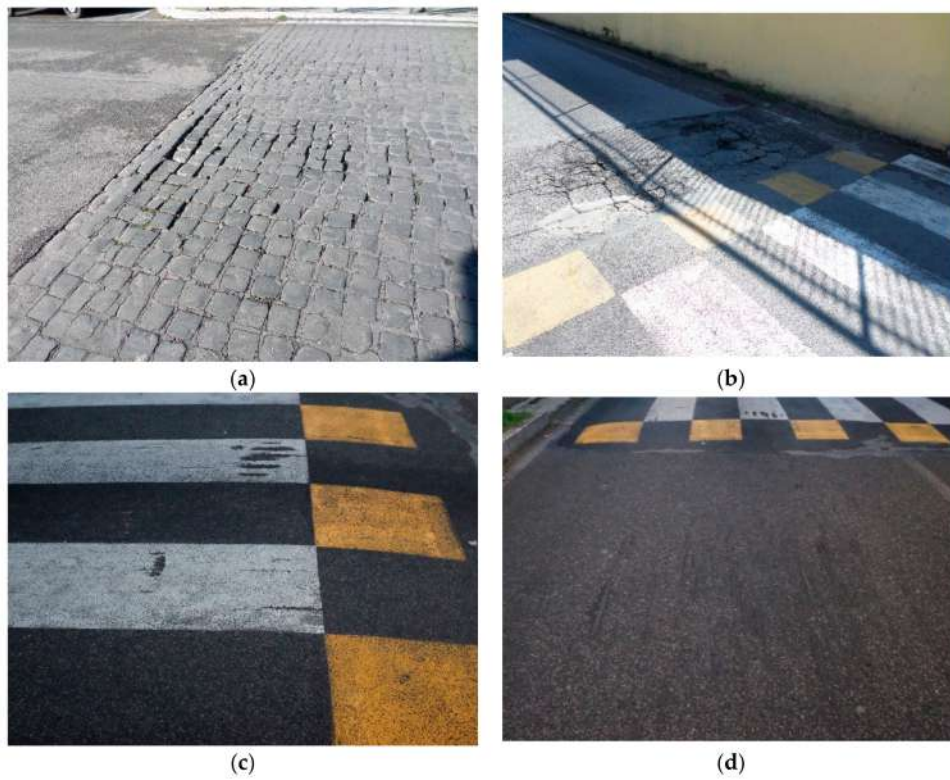
Figure 5. Example of surveyed distresses: (a) Depression on the access ramp; (b) depression after the exit ramp; (c) grooves on the pedestrian crossing surface; (d) grooves after the pedestrian crossing surface.
