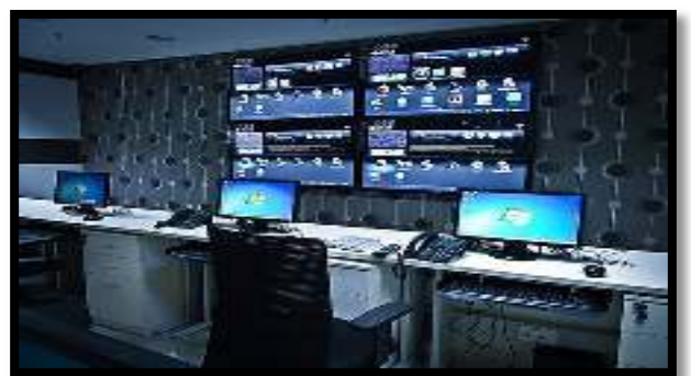
Gambar 7: Ruang kontrol/ monitoring
