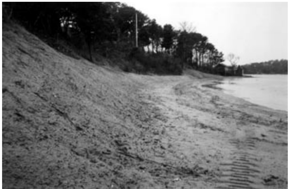
Fig 35. Fiber rolls covered with sediment
