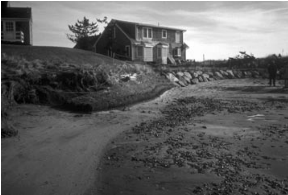
Fig 6. End scour on flanking erosion around bio-logs
