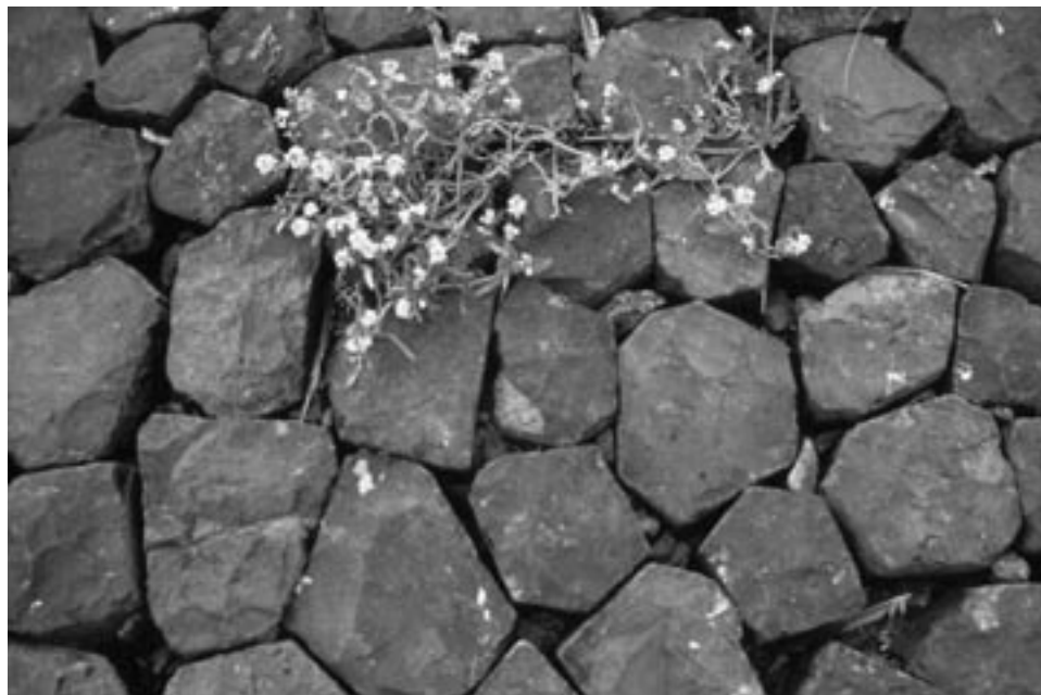
Fig 13. Vegetation growing through a rock revetment
