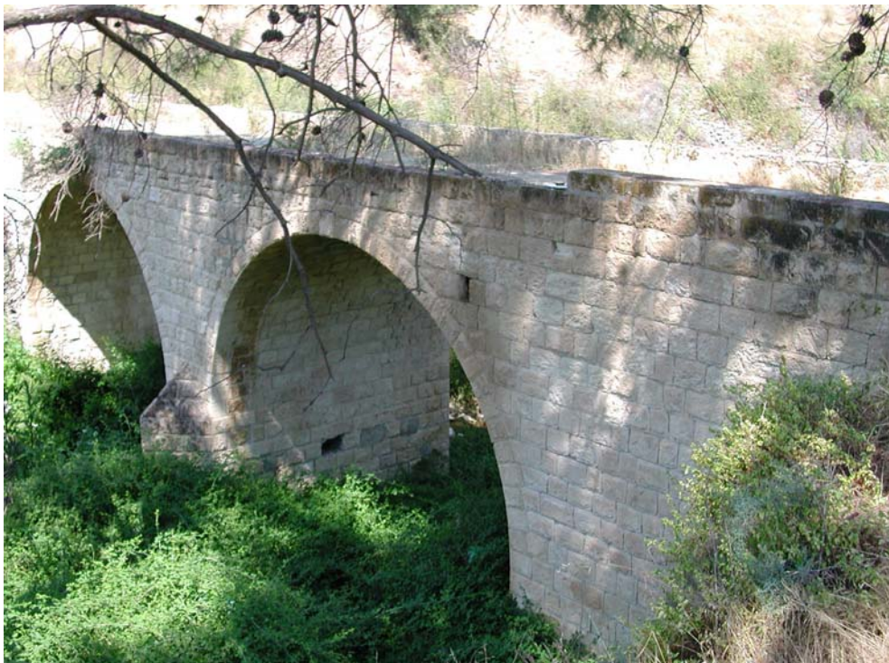
Figure 5.14: Atsas River Bridge with steep riverbank (photograph taken by Chris Parks - TAESP).
