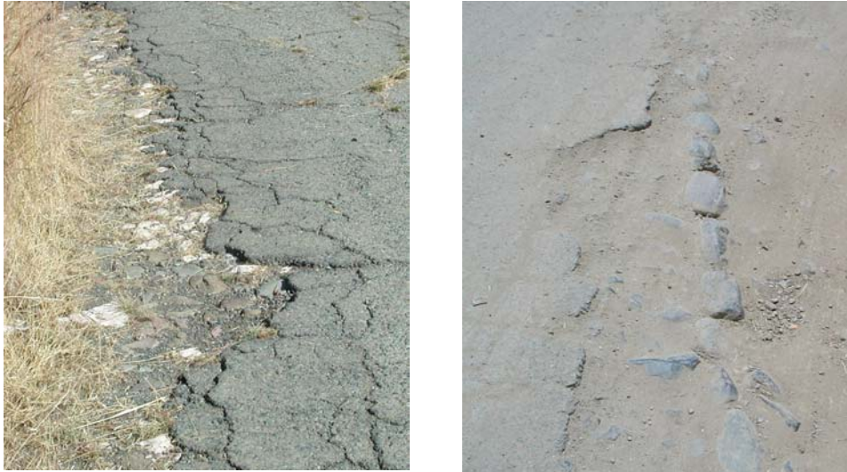
Figure 5.8: On left photograph of British Colonial road showing cobbling beneath a tarmac surface, on right view of road edging.
