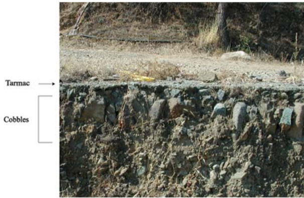
Figure 5.7: Cross section of British Colonial Road showing layering of tarmac and cobbling
