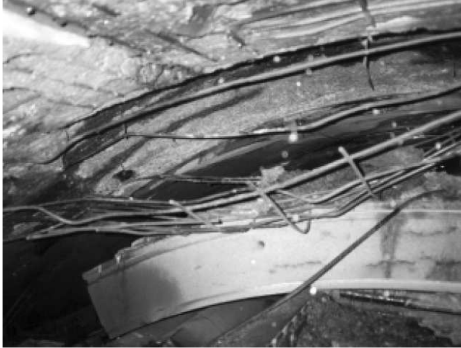
Figure 1.1.: The Great Belt tunnel lining damaged after the 1994 fire
