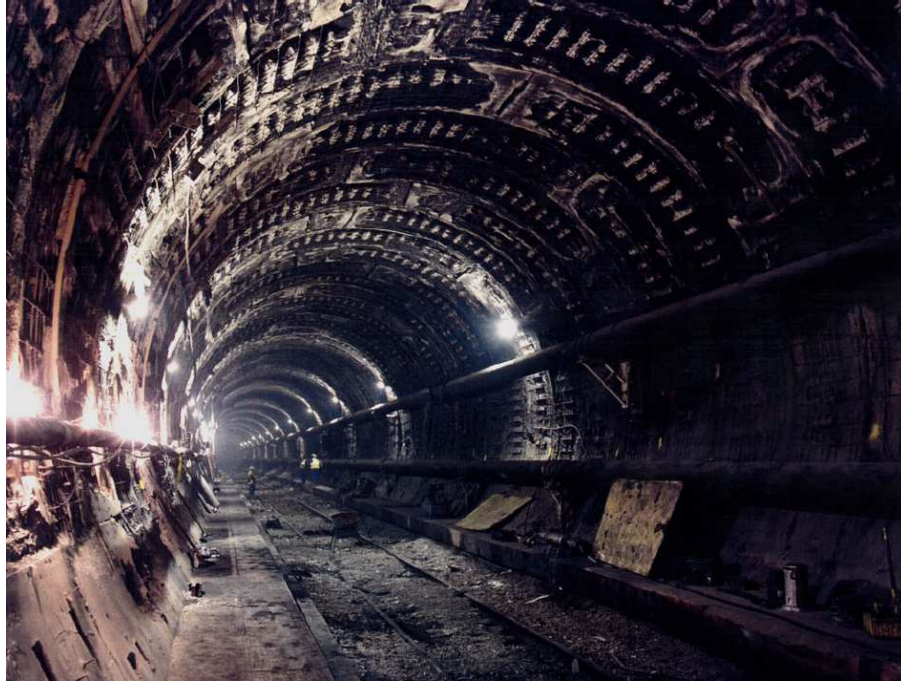
Figure 1.2.: Chanel Tunnel after 1996 fire
