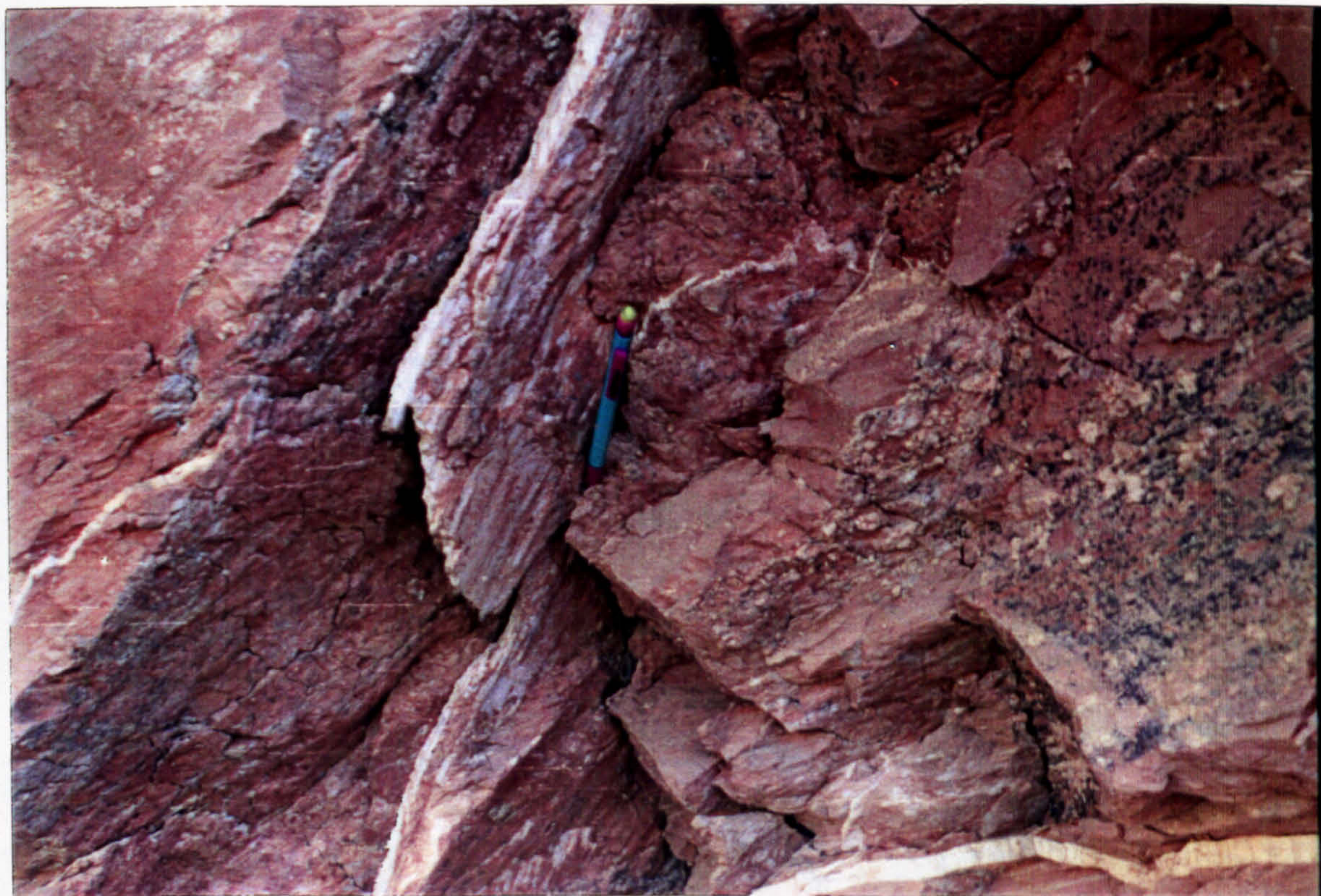
Fig. 7.8. Fault with oblique slickensides cutting the syn-rift Shihr Group rocks, north of Al-Hami area.
