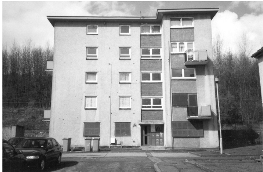
Figure 1 Ex-council flats with reported damp problems.
