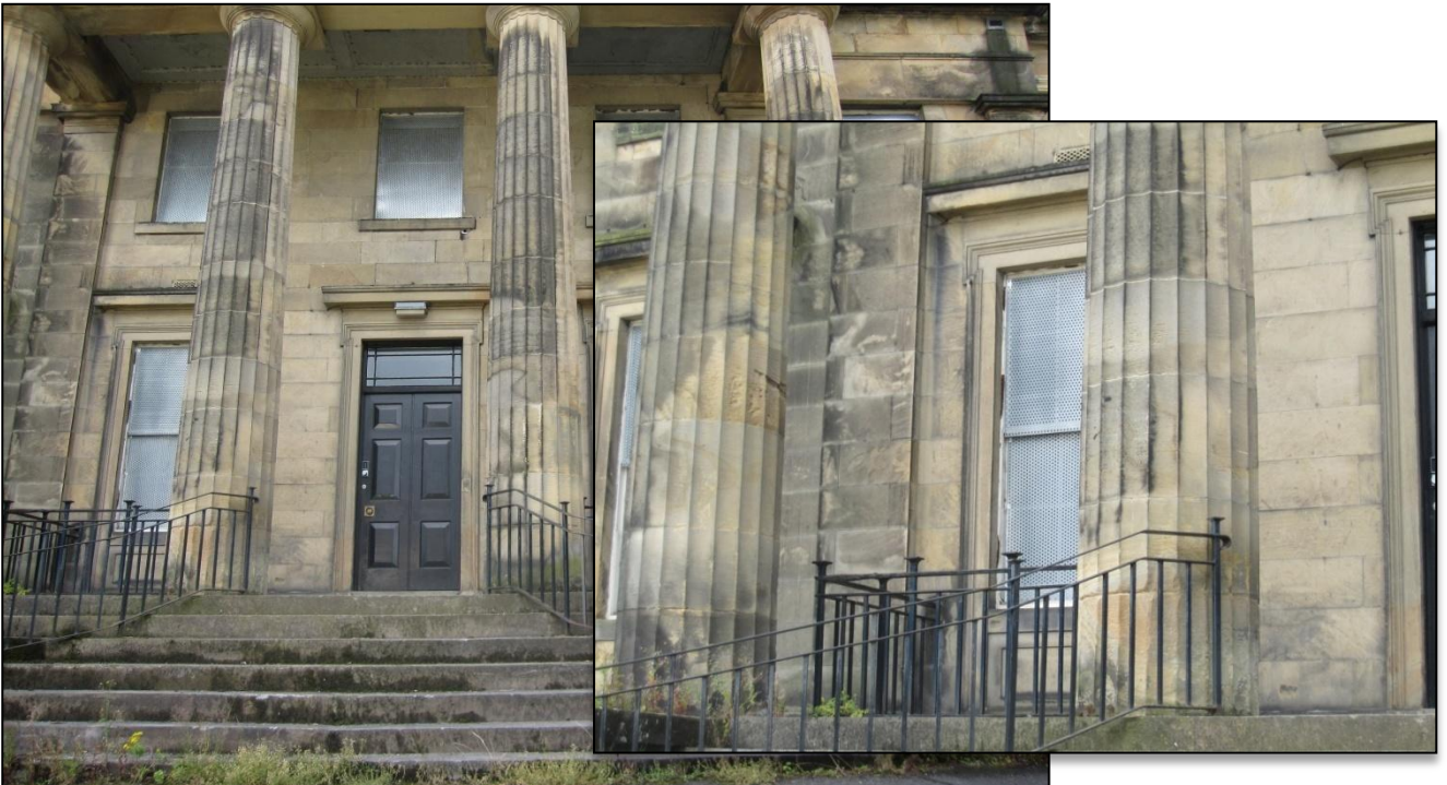
Figure 9: Former Commercial Bank front entrance colonnade, Spittal Street, Stirling. Disturbed bedding is visible in the ashlar and weathered columns of this former bank building. The building stone may be Thorneydyke Sandstone; further analysis would need to be undertaken in order to determine this.
