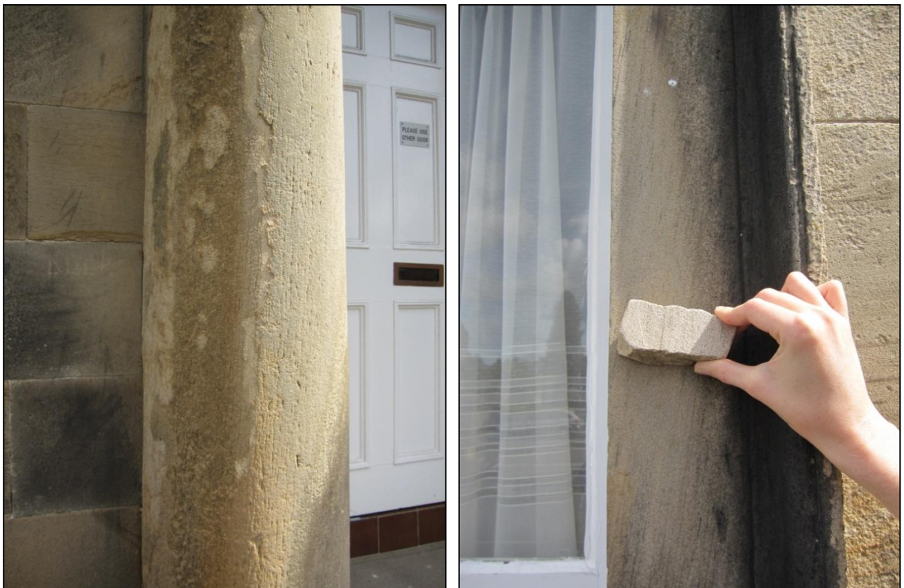
Figure 13: 19 Allan Park column (left) and window surround (right) alongside a sample taken from Drumhead Quarry. Laminated sandstone was very commonly used for paving and for columns and dressings. The sample of Drumhead Sandstone (right image) when compared to the sandstone dressings of 19 Allan Park has a very similar laminated appearance and colour.
