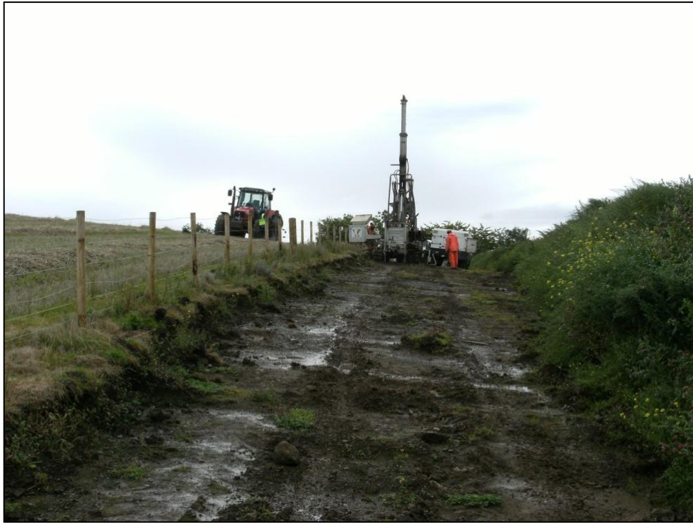
Figure 21: Drilling at borehole 09DH03P directly east of the currently exposed quarry face.
