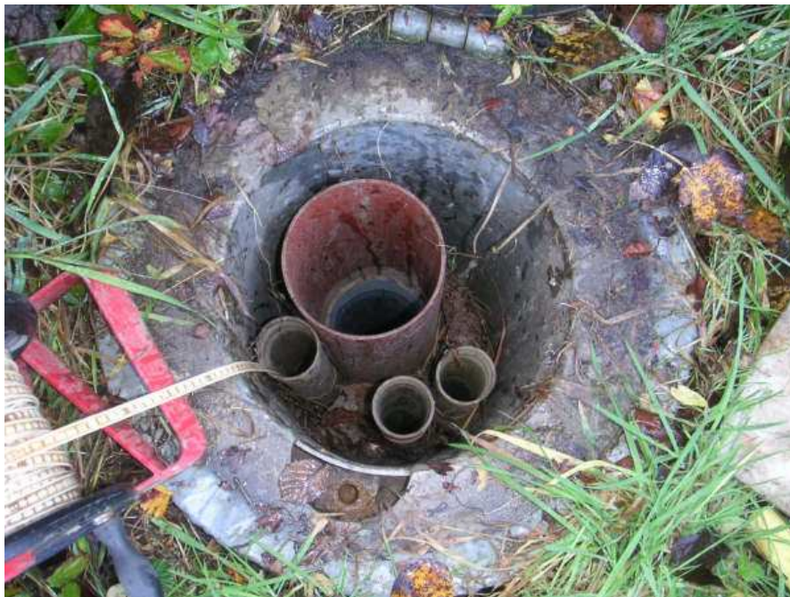
Figure 4.3. A typical piezometer nest installed by the Erftverband and RWE Power AG.
