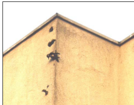
Picture 2. Woodpecker damage on the façade of a school in Neunkirchen, N.Ö. Source: Zottl
