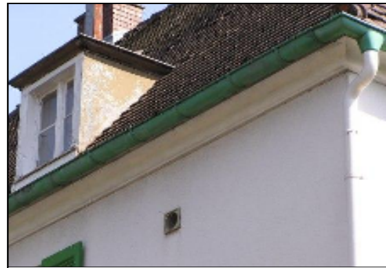
Picture 10. Example of the 'wall and roof dilemma' (Freiburg). To attach 16cm of insulation requires the roof to be rebuilt.
