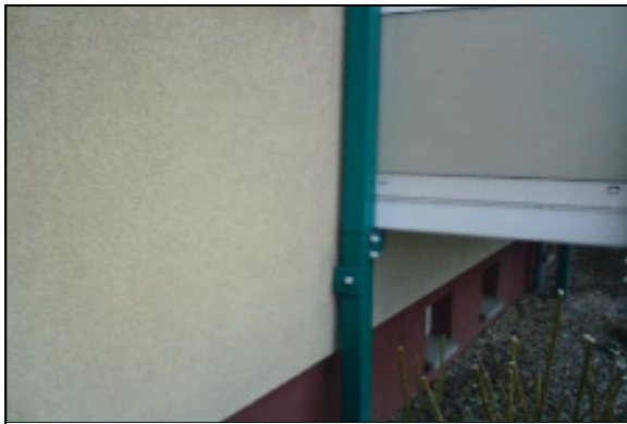
Picture 9: A de-coupled balcony attachment on the communist-era apartments in Picture 8.
