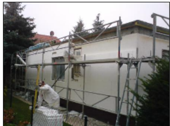
Picture 4: 8cm of external wall insulation being (illegally) applied to a house extension. The legal minimum requirement is 16cm.
