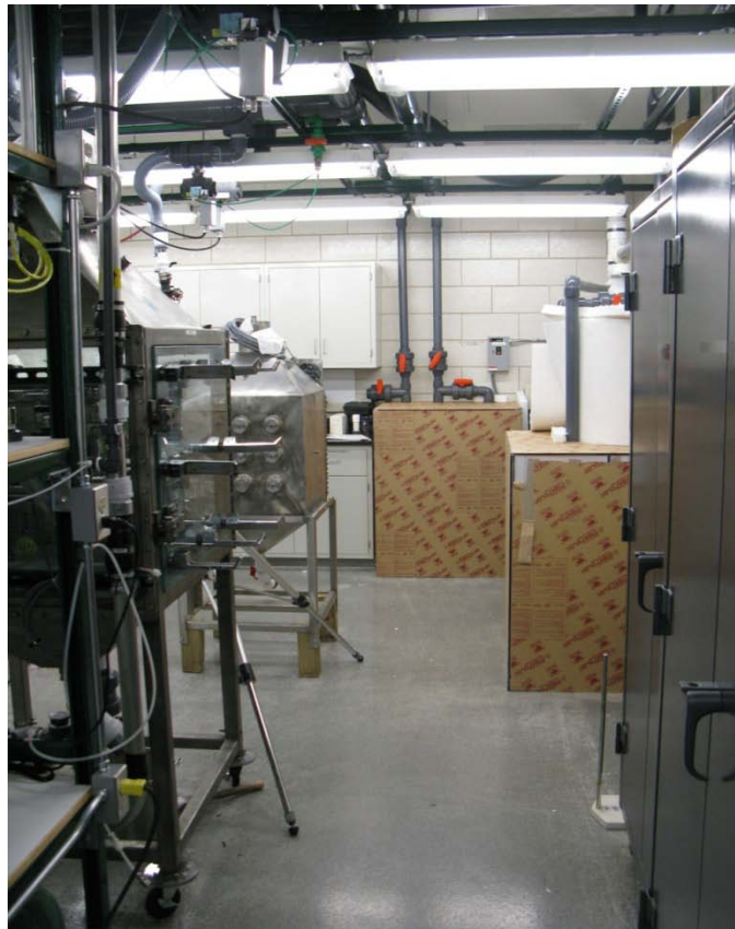
Figure 12. View of acoustical enclosures surrounding air compressors
