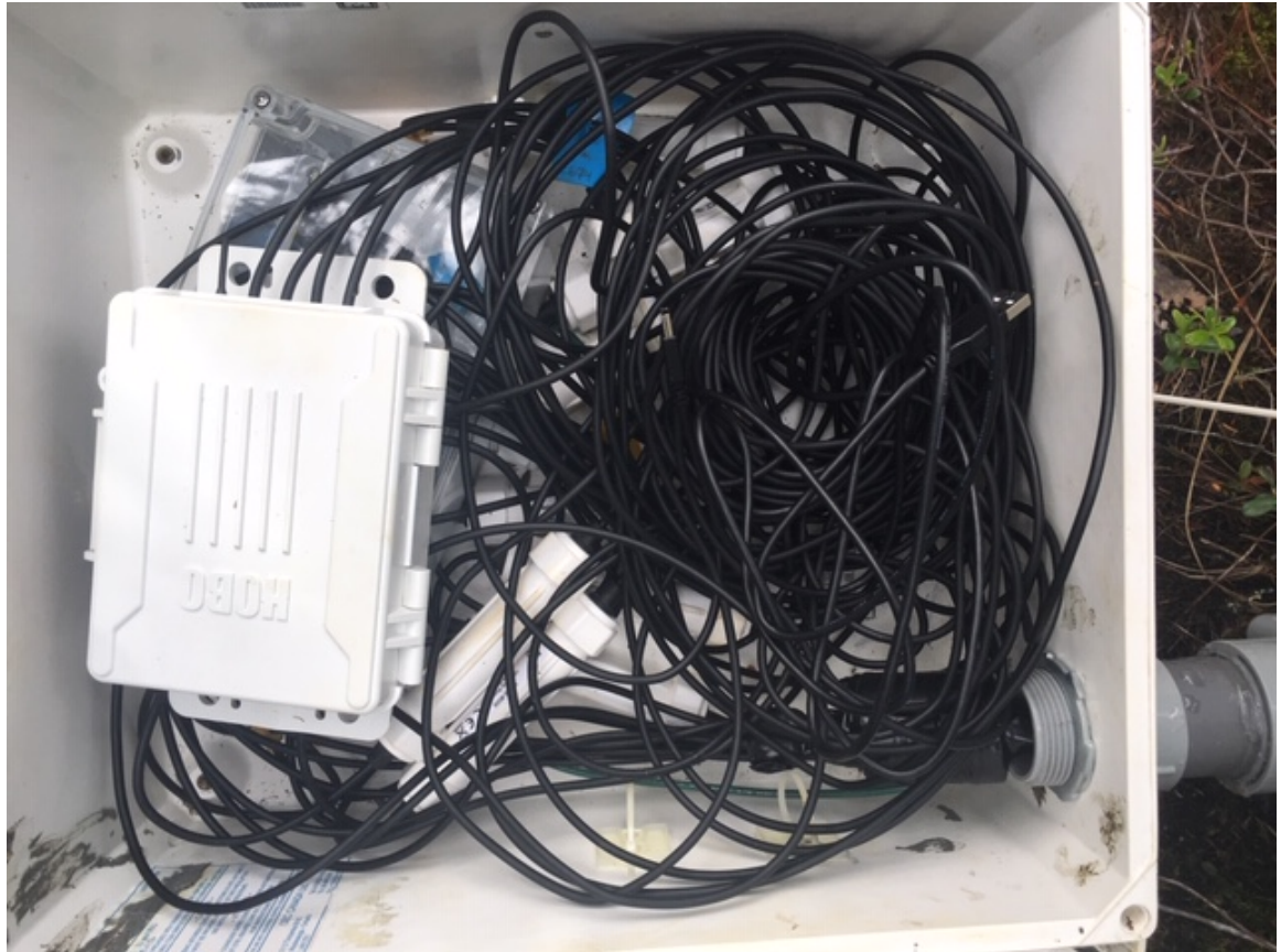
Figure 3.14: Station Two Instrument Housing
