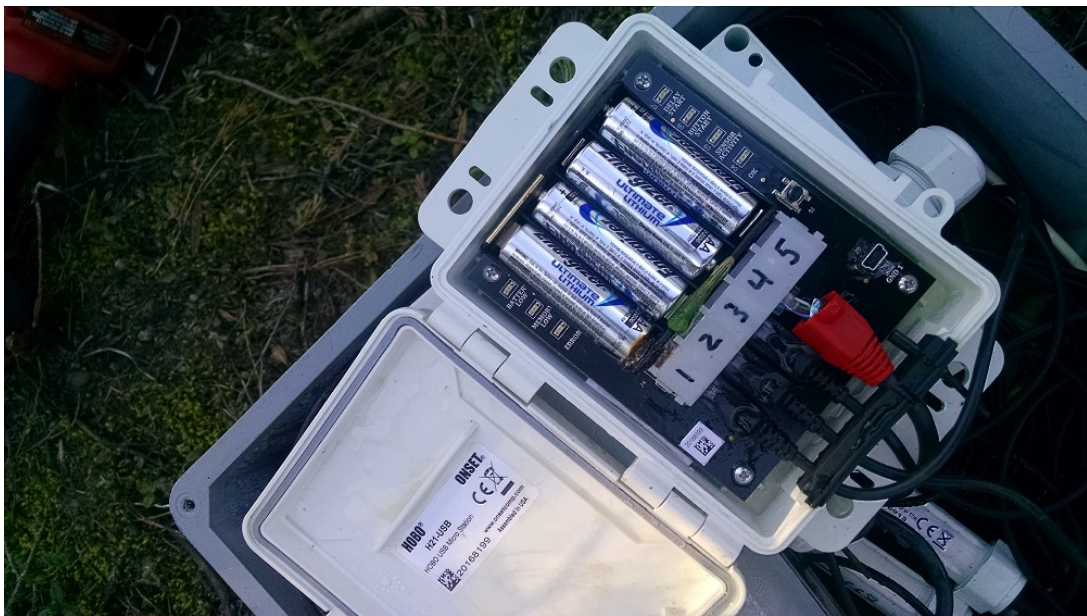
Figure 3.11: Data Logger Damage from Corrosion
