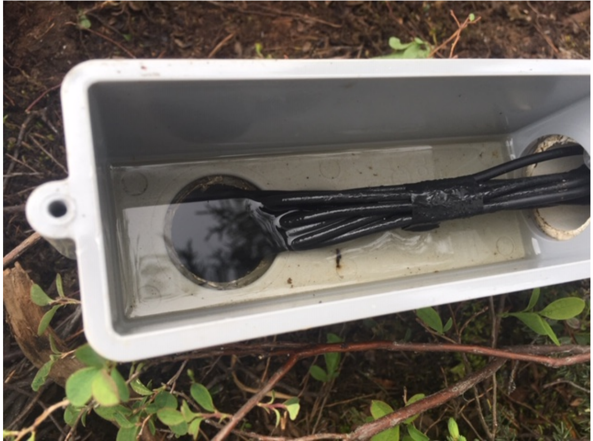
Figure 3.9: Borehole One Flooded
