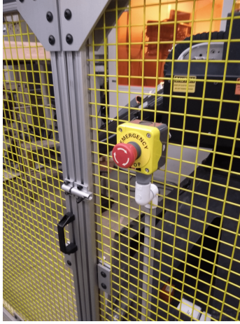
Figure 12. Emergency button on MTA safety fence
