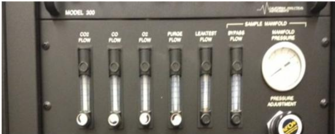
Figure A.4: CAI flow meter panel
