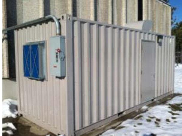
Figure 3.23: Ingersol Rand H50A-SD Compressor trailer located outside the COAL Lab
