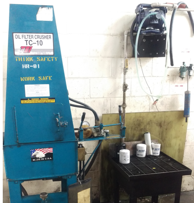
Figure 2 - Waste Motor Oil Collection Area with Filter Crusher
