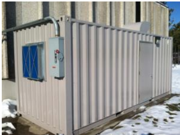
Figure 26. Ingersoll Rand H50A-SD Compressor installed outside COAL Lab
