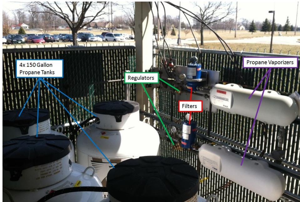
Figure 34. Propane tanks and Zimmerman LPG propane vaporizers
