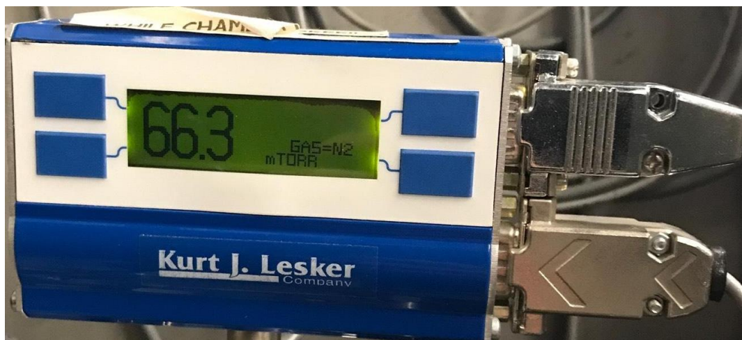
Figure 3.10: Pirani Pressure Gauge that Controls Crossover to Cryopumps
