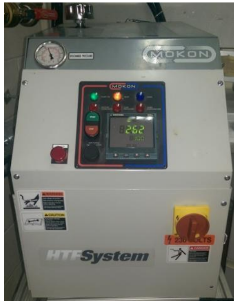
Figure 3-23: Mokon thermal management system
