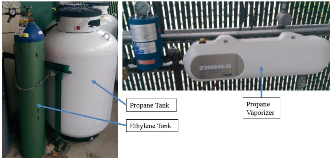
Figure 3-22: Propane and Ethylene tanks (left), propane vaporizer (right)
