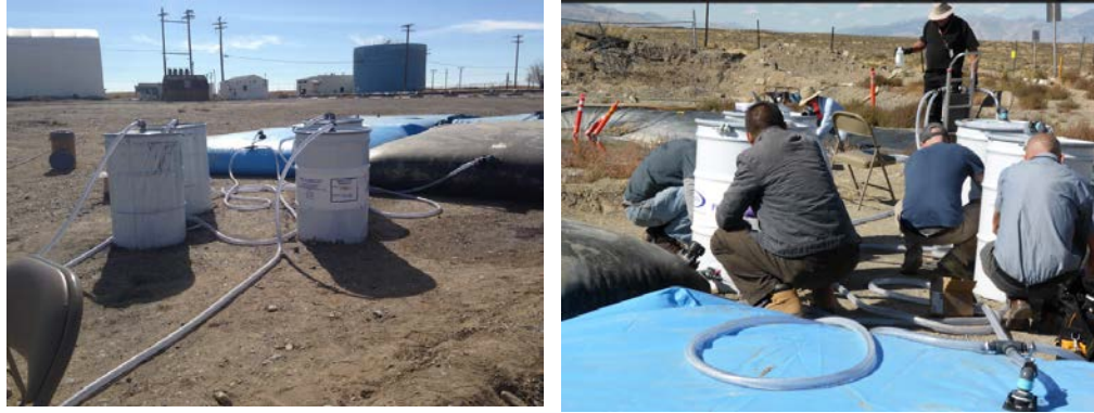
Figure 13. Flowsorb® drums filled with GAC, and sampling during Field Scale experiment (Left to right)
