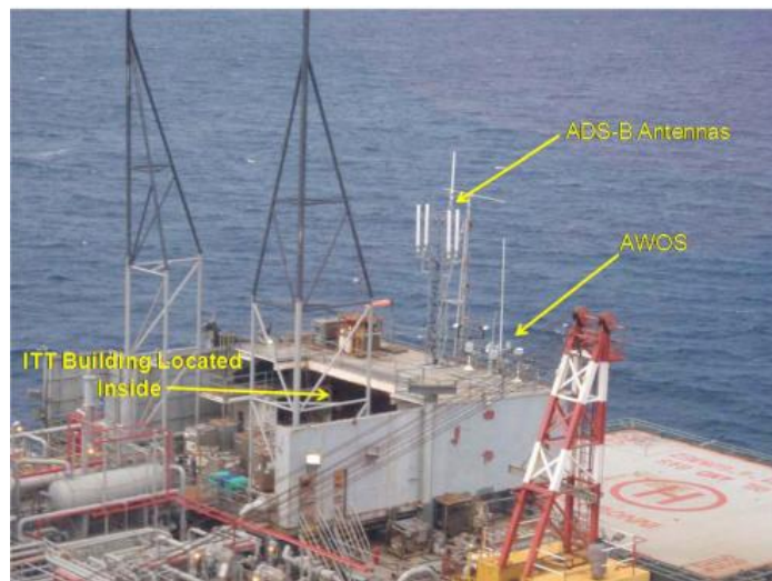
Figure 7 - ADS-B equipment aboard an oil rig [37]
