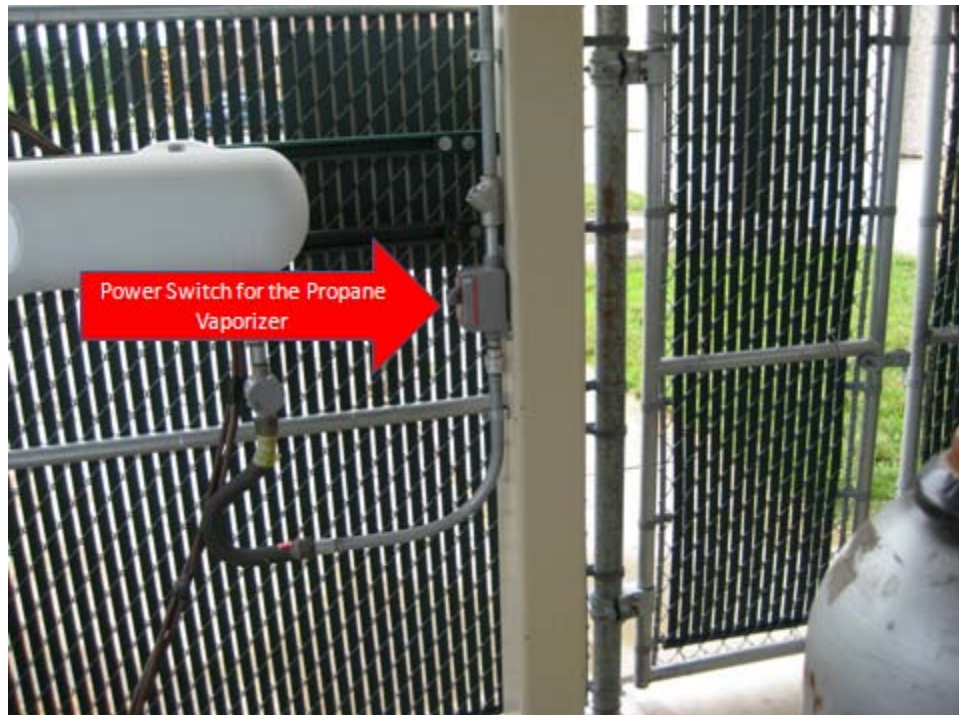
Figure A.14: Showing location of the power switch for the Vaporizer inside the Tank Farm.
