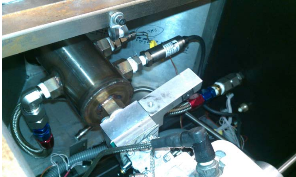
Figure 20: New 3 inch stainless pipe used as an intake manifold
