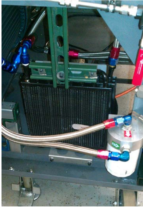
Figure 21: New oil cooler installed to reduce compressor oil temperature
