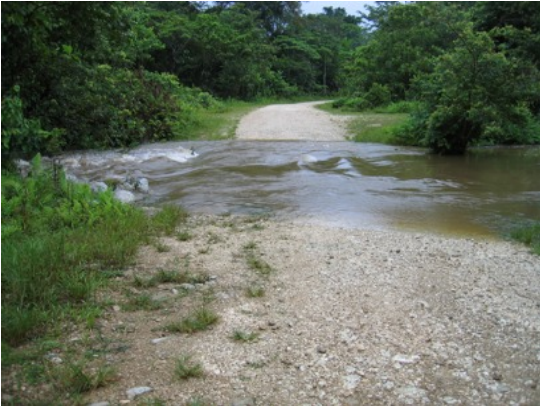
Fig. 19 Unsealed Roads are Subject to Flooding
