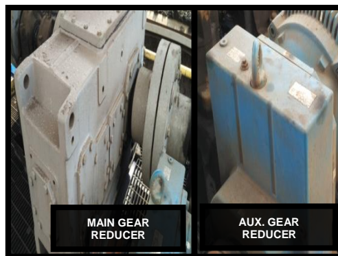
Gambar 2.7 Main dan aux gear reducer Submerged Scrapper Conveyor ( Sumber : Dokumen foto PLTU Unit 1 & 2 ) 2.2.6 Programmable Logic Control (PLC)
