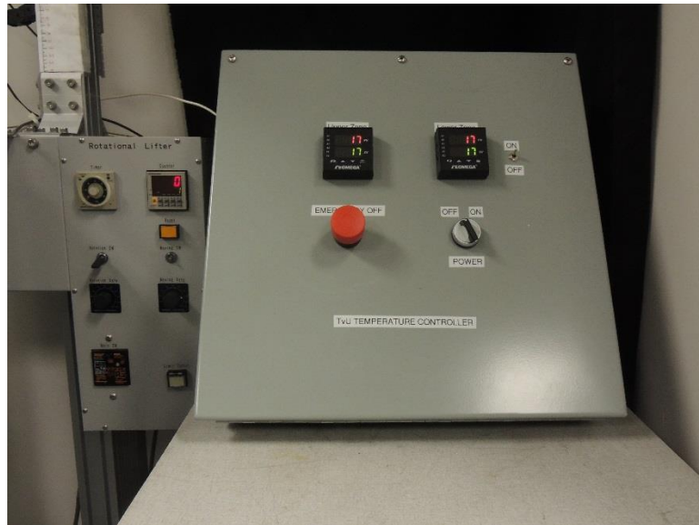
Figure 66. PID temperature controller
