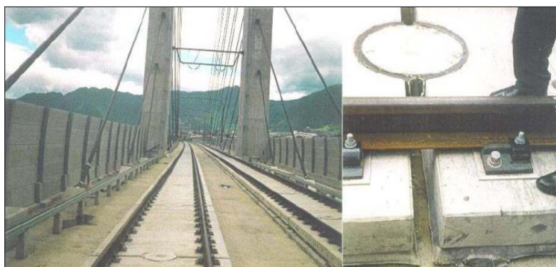
Figure 4. A sample of implemented Shinkansen slab track [46]
