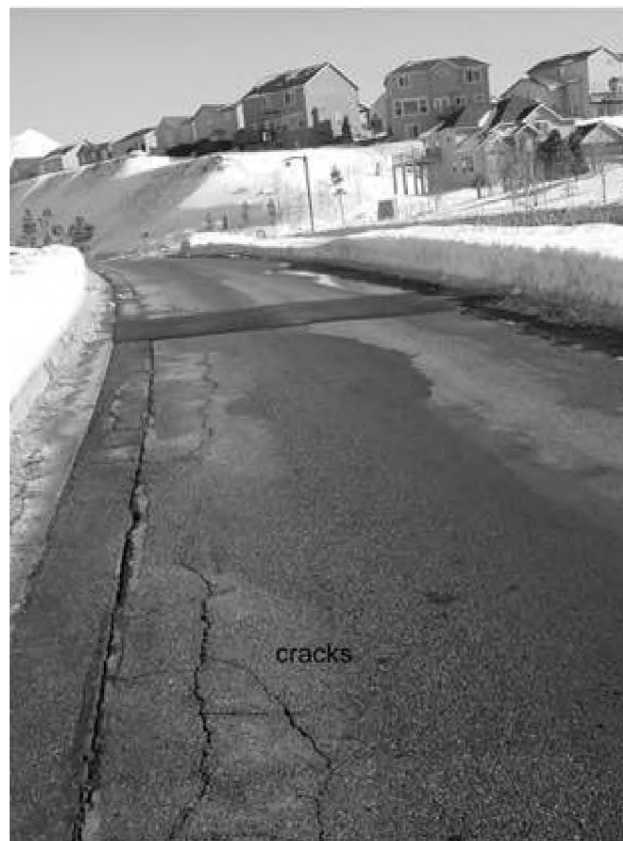
Figure 11. In the background, houses have been built upon a terrace above a head scarp. In the foreground, radial growth cracks indicate that local failure zones are setting up in the asphalt along Deer Ridge Road where the road runs along the ridge top, which is the crown of the LVL. For reference, the LVL is to the left of the photograph taken.
