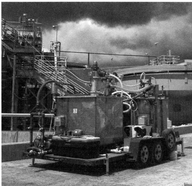
Figure 1 — Mobile ASH system installed at Midas.
