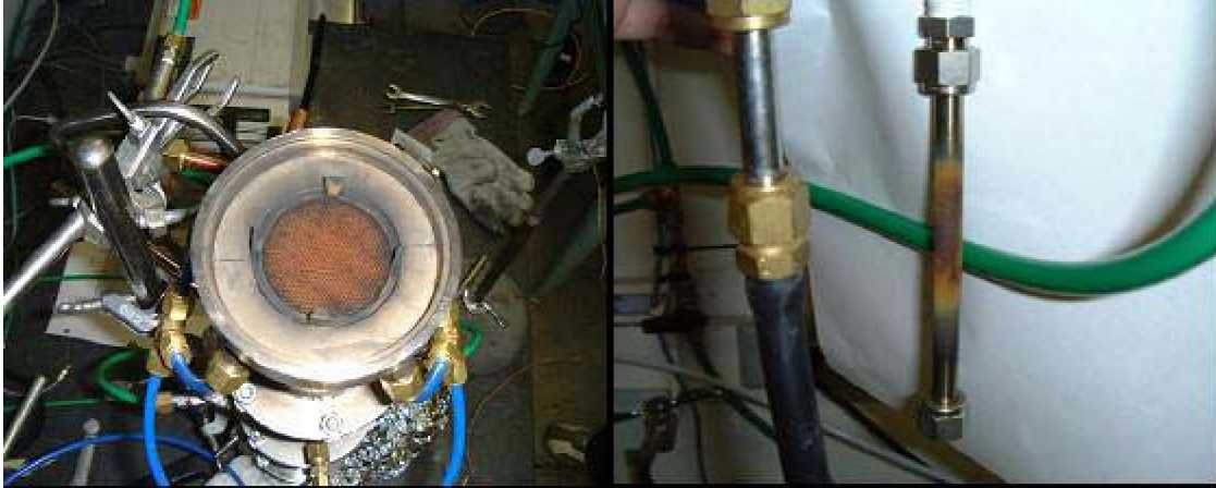
Figure 35. Second-stage burner (left) and sampling probe (right), showing iron oxide deposition.
