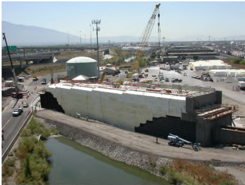
Figure 1.1. Typical freestanding EPS embankment (Utah Transit Authority Light Rail System, Salt Lake City, Utah)
