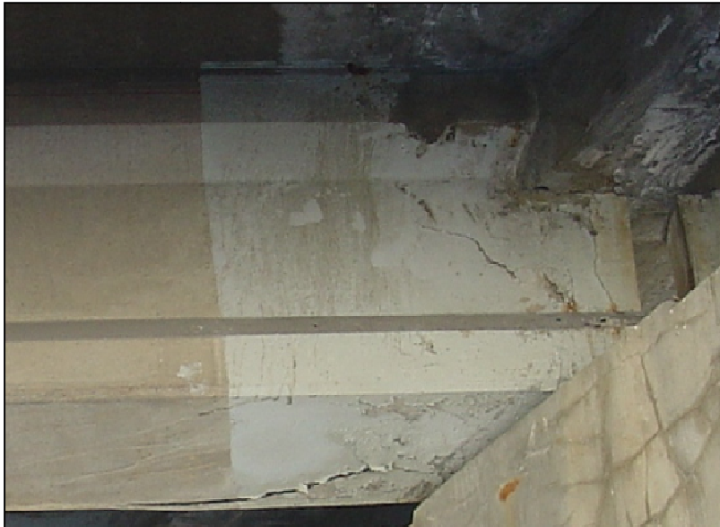
Fig. 4.1 – Girder end damage with diagonal cracking
