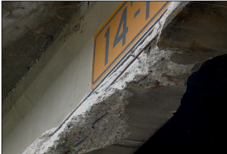
Fig. 5.1 – Girder damage from vehicle impact
