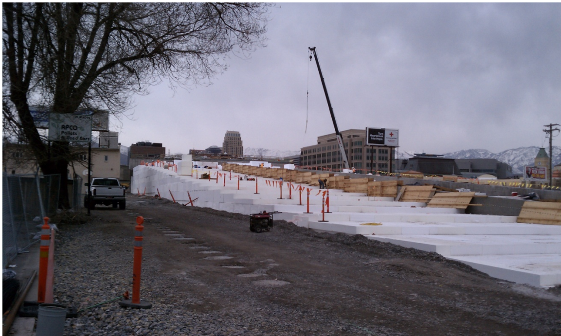
Figure 4: Recent viaduct construction project in Salt Lake City, Utah implementing EPS geofoam as soil replacement.
